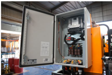
Separate fuse and controller box for organized and efficient electrical management
