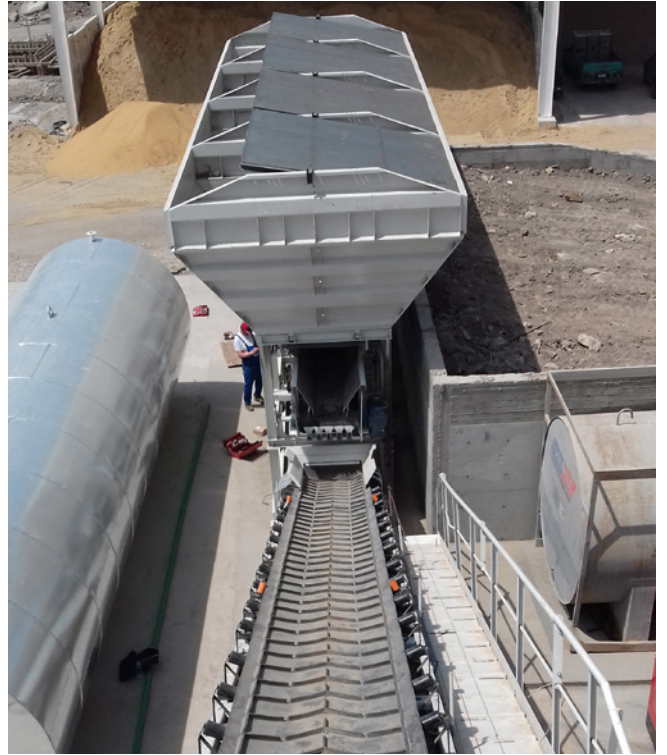
Inclined conveyor with one side walkway
