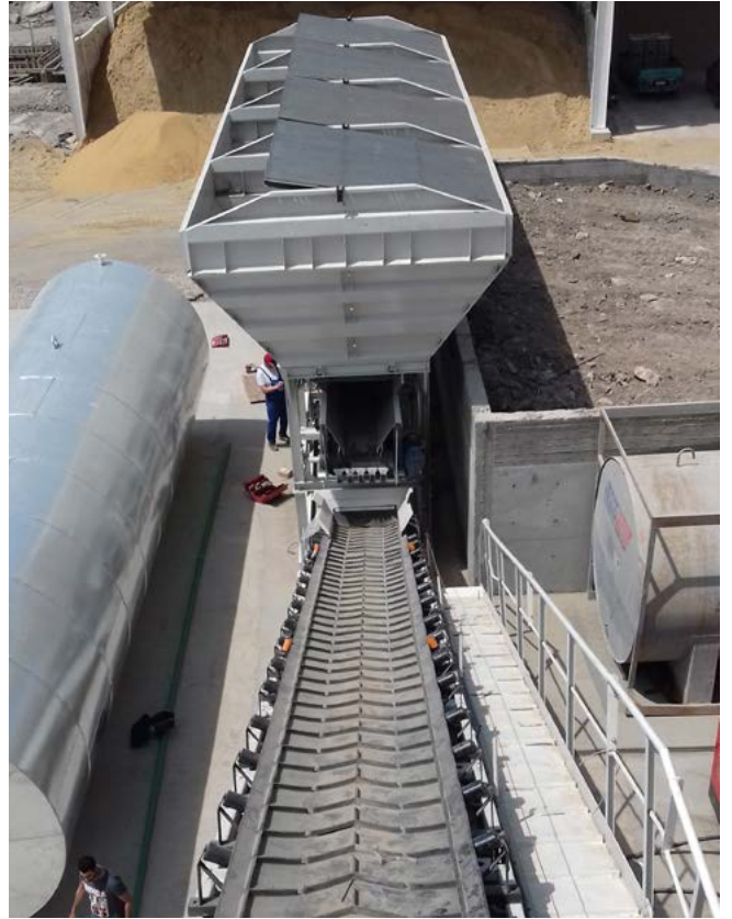
Inclined conveyor with one side walkway.
