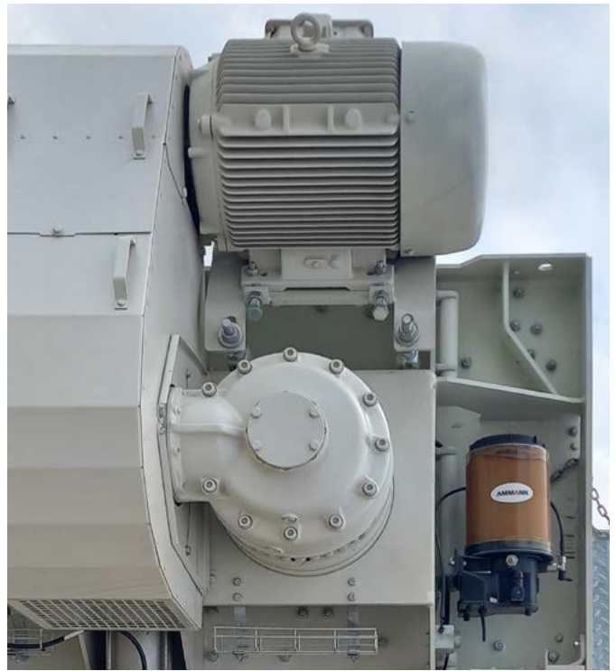
Mixer drive with automatic central greasing system.
