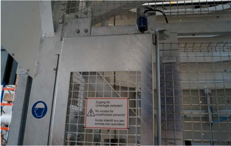
Access area secured through limit switch according to UVV.
