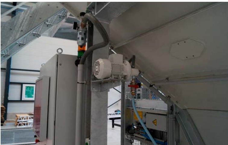
Optional additive dosing by powerful dosing pump.
